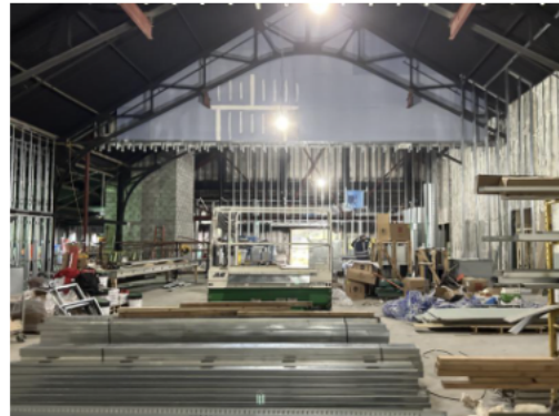
A new second-story space has been added above what will be the aquatic center.
