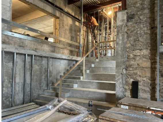
In the west lobby of the Montauk Playhouse, a new staircase and stadium-style seating are being built. Denis Hartnett Photos
